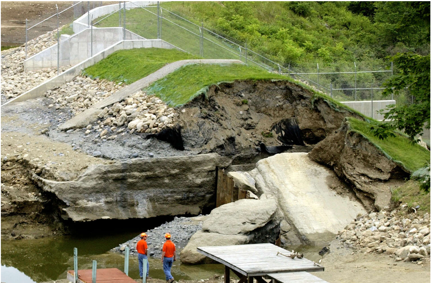
New York State Department of Transportation workers look over the dam area on the south end of Hadlock Pond in Fort Ann on July 7, 2005. The dam gave way earlier that month. Paul Buckowski / Times Union
