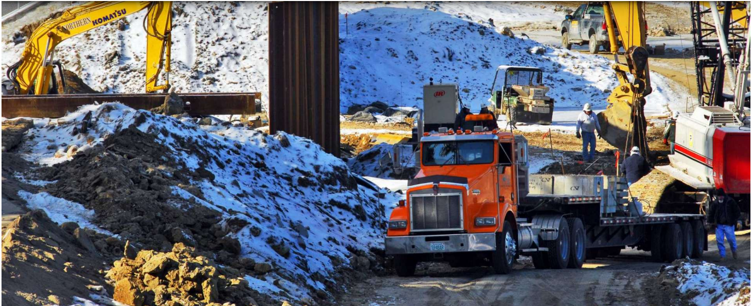
Workers reconstruct the Hadlock Pond Dam on Jan. 17, 2007, in Fort Ann. Town Supervisor Sam Hall says the town has had the rebuilt dam inspected annually even though it's not required. John Carl D'Annibale / Times Union
